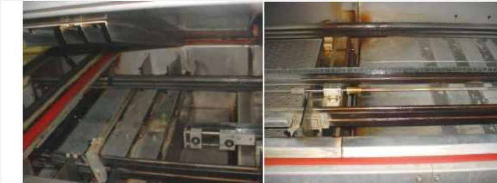
Manual cleaning of reflow oven: before
