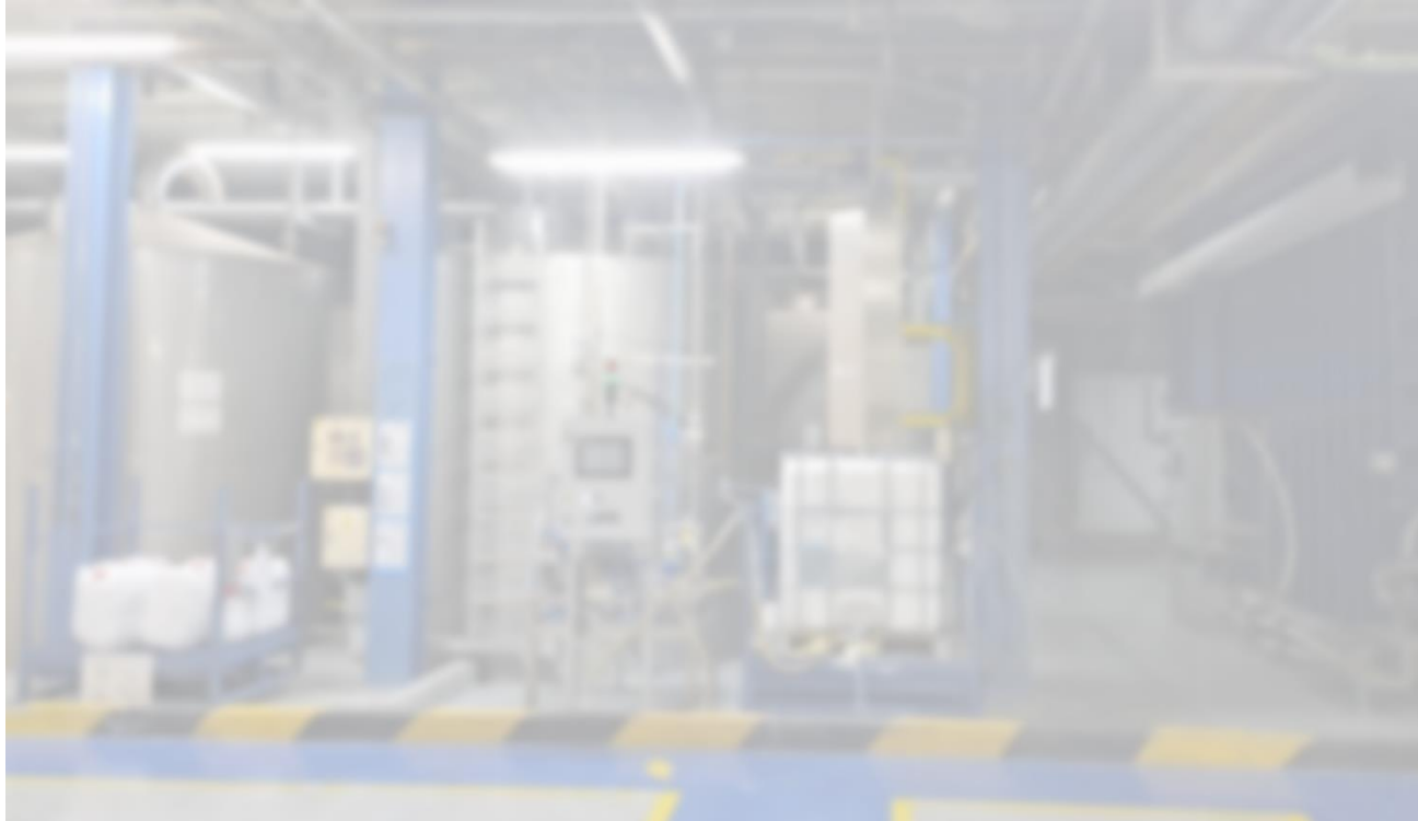
AREA TO CHARGE CHEMICAL PRODUCTS (DOSAGE AUTOMATION)
